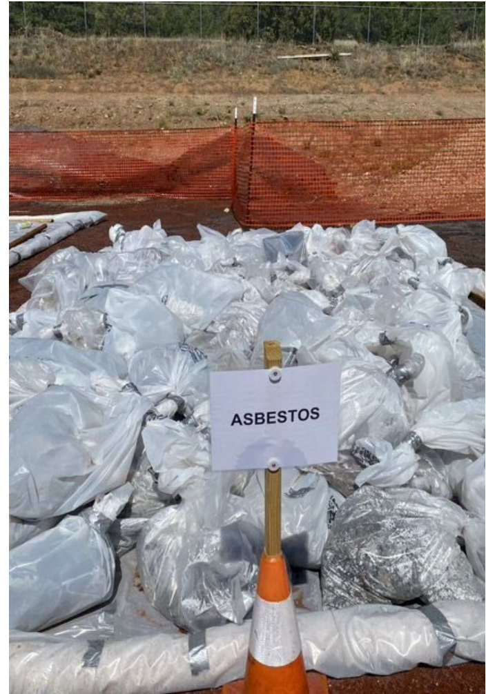
Picture 2: Waste (asbestos) at the Staging Area
